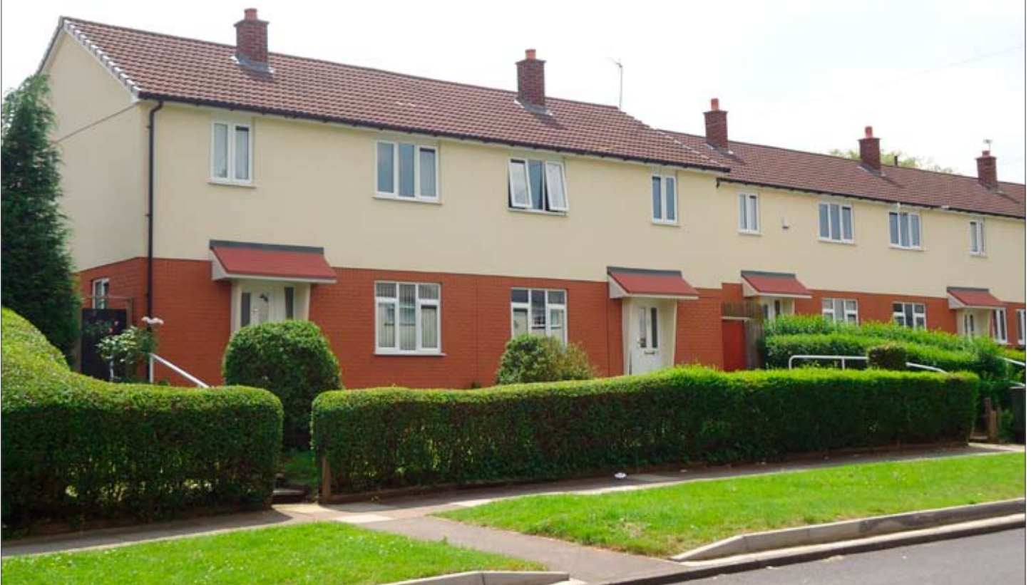
Airey semi-detached properties after refurbishment showing Macerend brick effect render to ground floor and Acrylic render to first floor.
